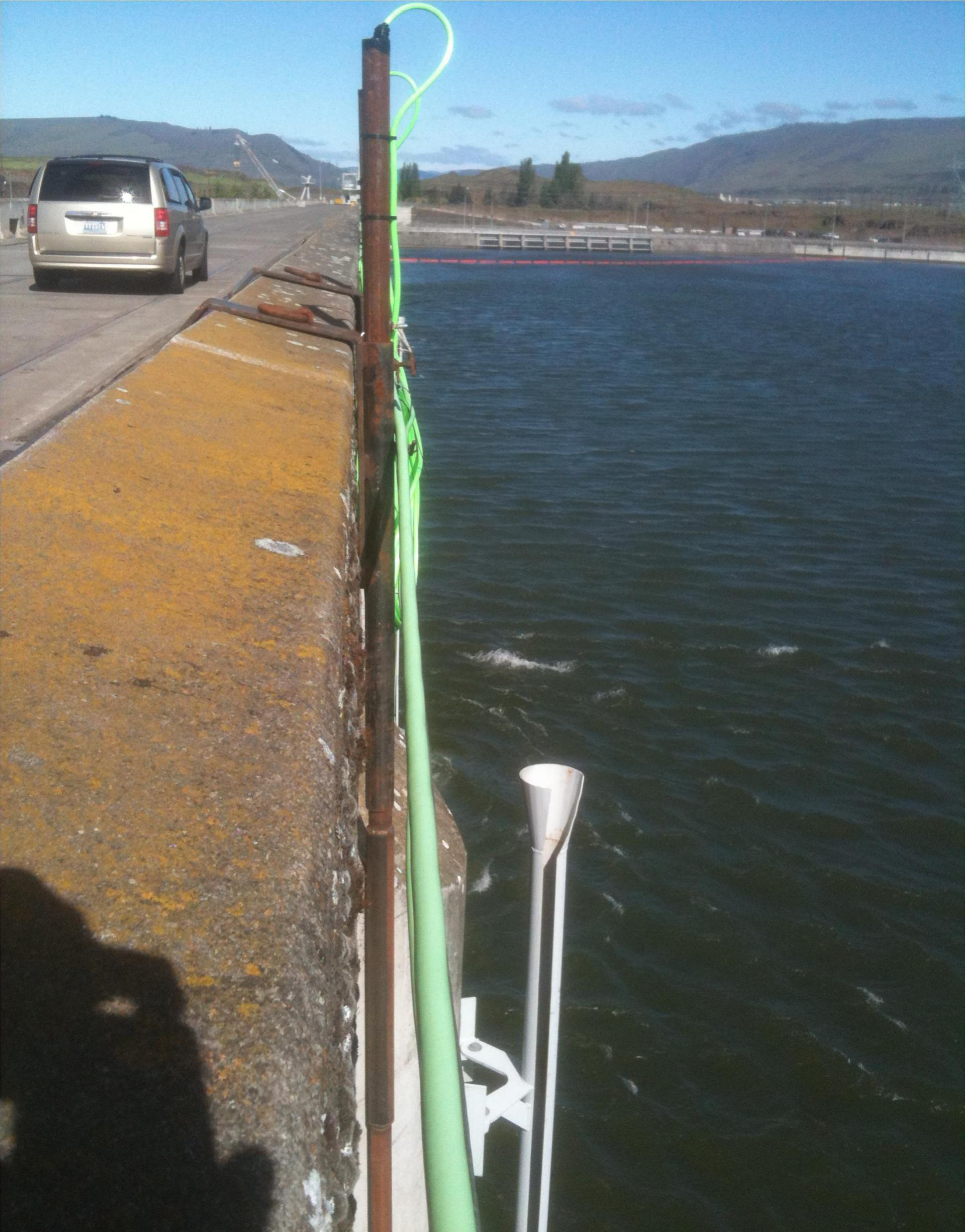
Battelle's transducer failed on spillway pier nose between 9 and 10; TDS installed shallow pipes with hydrophones in place to maintain data collection.
